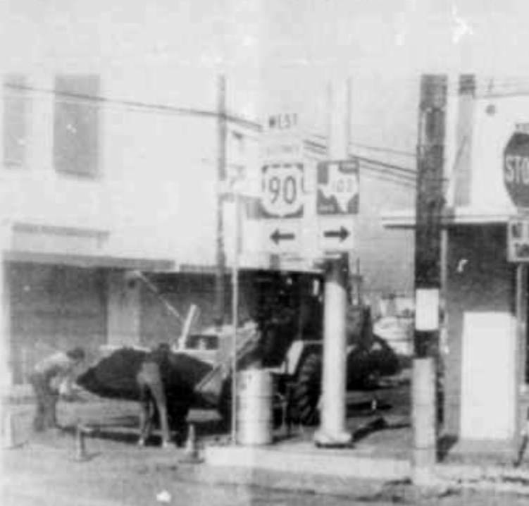
That bump you should remember if you ever drove down West Main street has disappeared. Last week city crews graded the bump in the concrete and filled the hole with asphalt. The work was just one of the many improvements which have been made in city streets in conjunction with the street program approved by voters a year ago.
